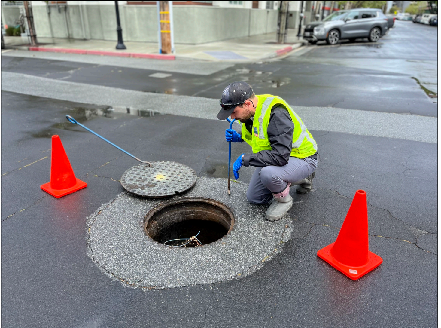
Vector Control Technician Devon MacDonald inspecting a sewer manhole for rodents in downtown Redwood City.
